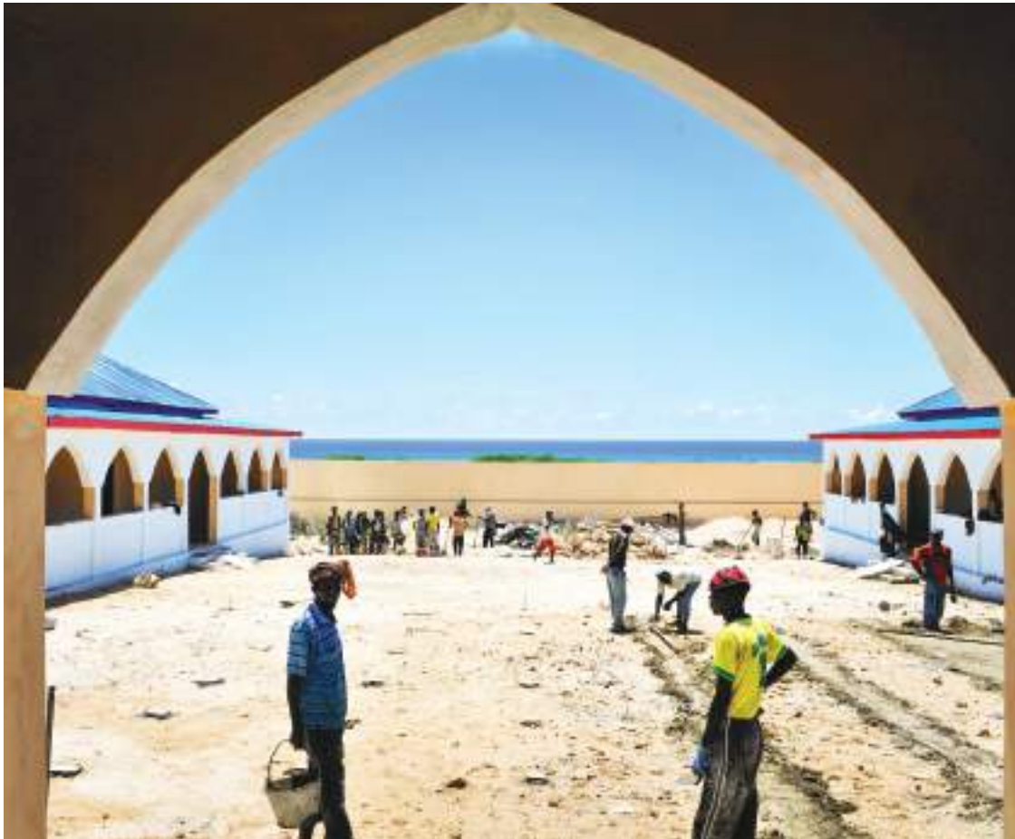
Construction work ongoing at the Mohamud Hilowle Primary and Secondary School in Mogadishu. The school was constructed with funds from AMISOM - 21 October 2012
